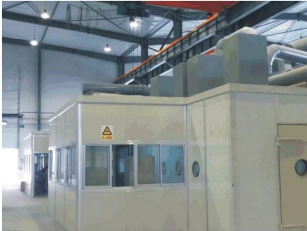
进口喷涂房及喷砂房 Spray and blasting room
